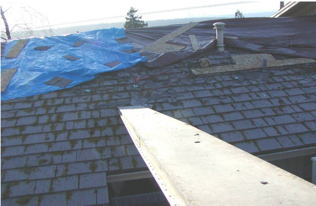
Photo 2: A view of the plank and roof at the incident site from the truck bed.
