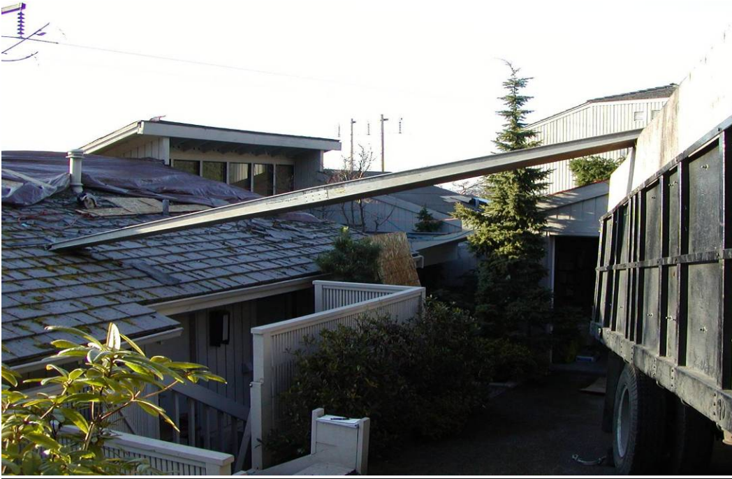
Photo 1: The job site after the incident, showing the plank from the roof to the edge of the truck bed.
