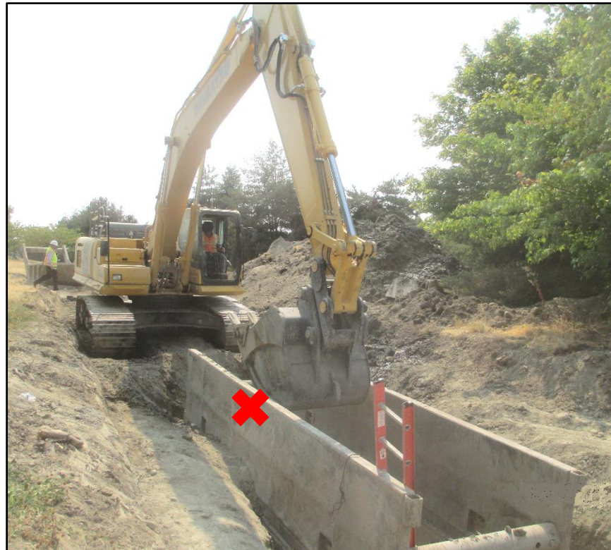
Photo 1. Excavator with bucket in its approximate position when it pinned the spotter against the top of the trench box.
