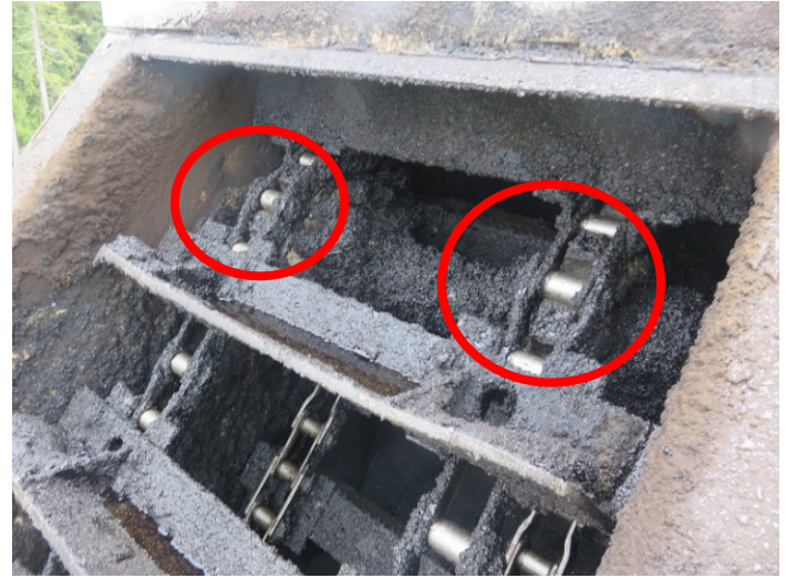
Photo 7: Conveyor gearbox with asphalt buildup on slats, drag chain, and head sprockets (circled) located under the drag chain. Workers use a pneumatic chisel to remove the asphalt from the sprockets so that they could remove and replace them.
