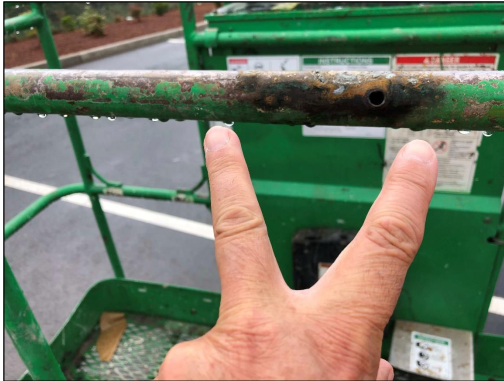
Photo 1. Entrance location where electric current made contact on railing of boom lift basket after arcing from a power line.
