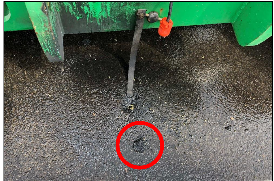
Photo 3. Hole burned into asphalt by electrical current (circled).
