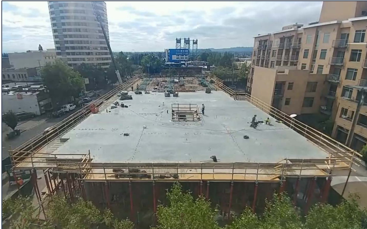
Photo 3. Security camera image of the building's second floor deck prior to the fatal incident. The stairwell opening with guardrails around it is in the center of the photo.
