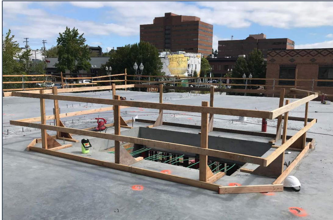
Photo 1. Stairwell opening the framer fell through.
