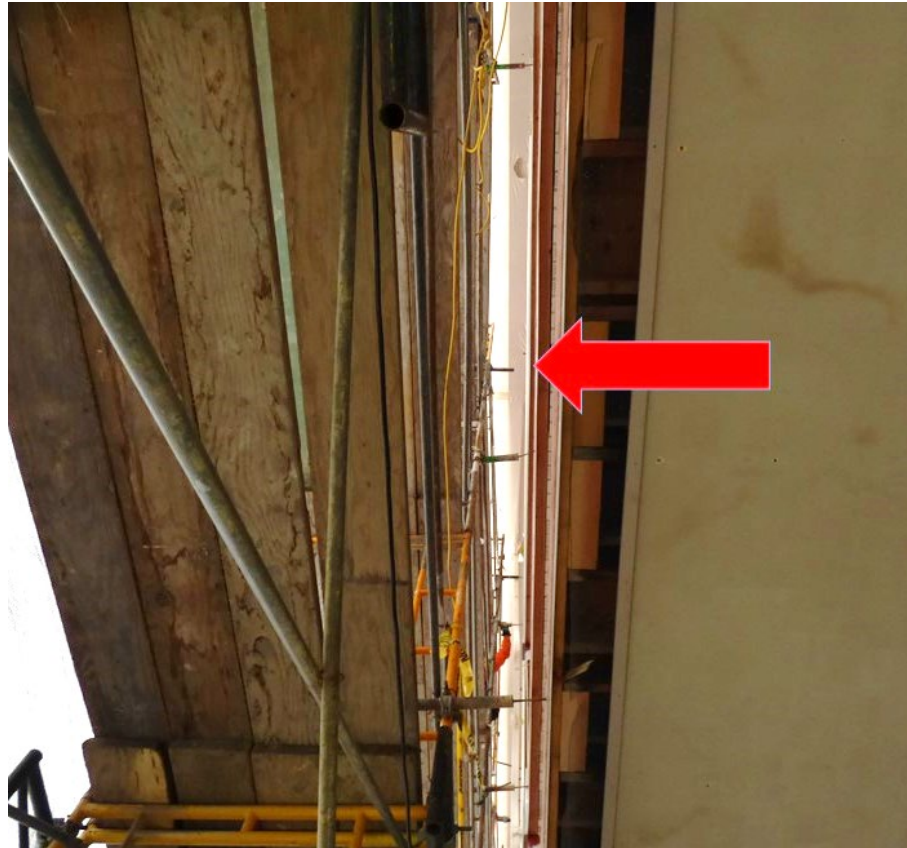
Photo 2. View from below the 12 ½-inch gap between the building and the scaffold (indicated by arrow) where the laborer fell through.
