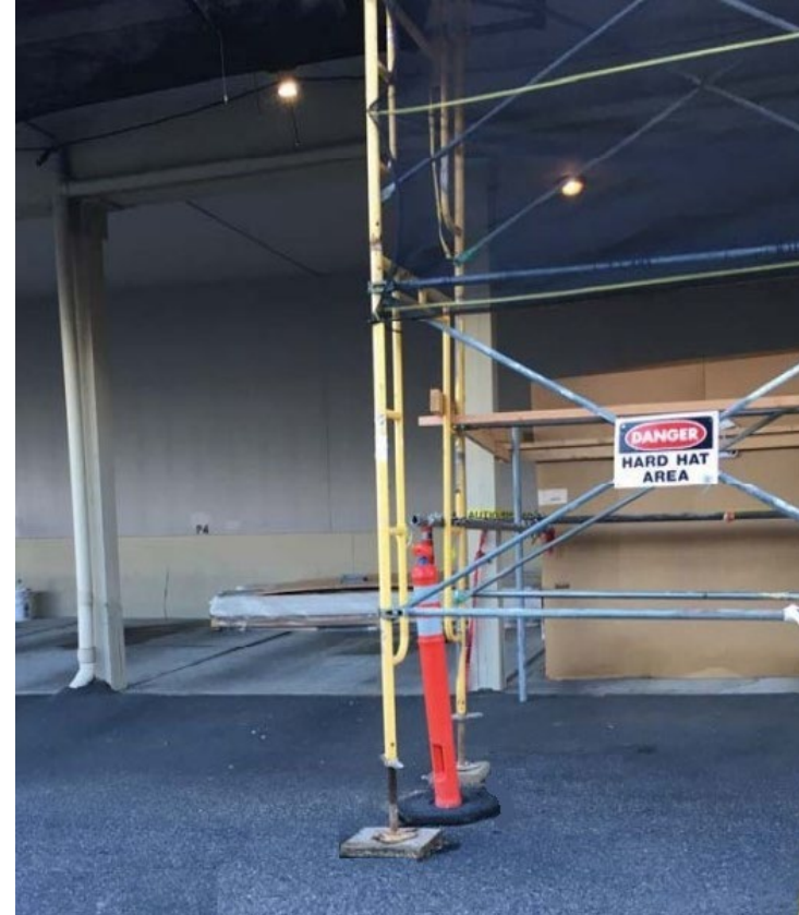
Photo 4. Location where the laborer landed after falling 25 feet from the scaffold cross braces.
