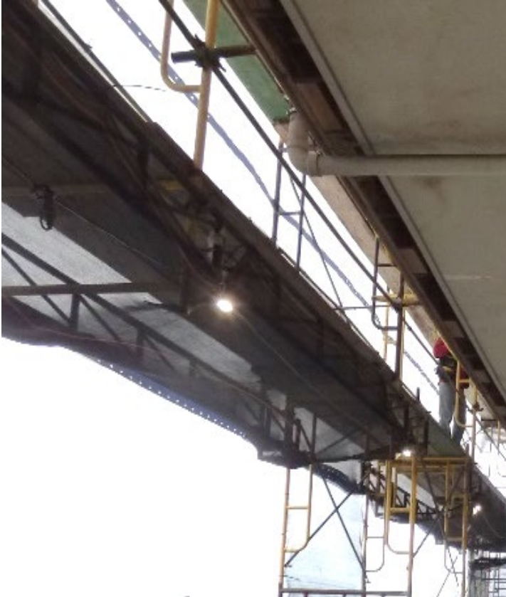
Photo 3. View from ground level showing cross braces and position in relation to the building.
