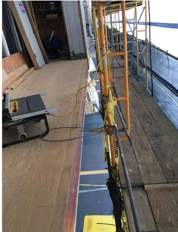
Photo 1. The 12 ½-inch gap between the building and the scaffold where the laborer was climbing the scaffold cross braces when he fell.
