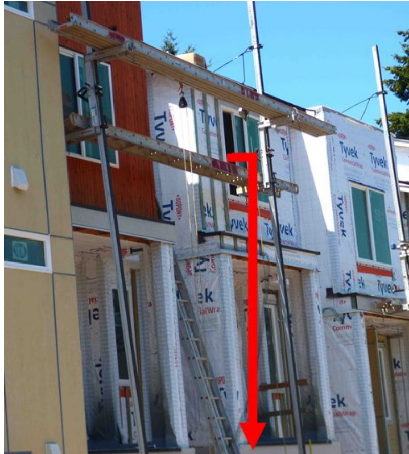
Photo 1. Unguarded pump jack scaffold from which the installer fell 23 feet.
