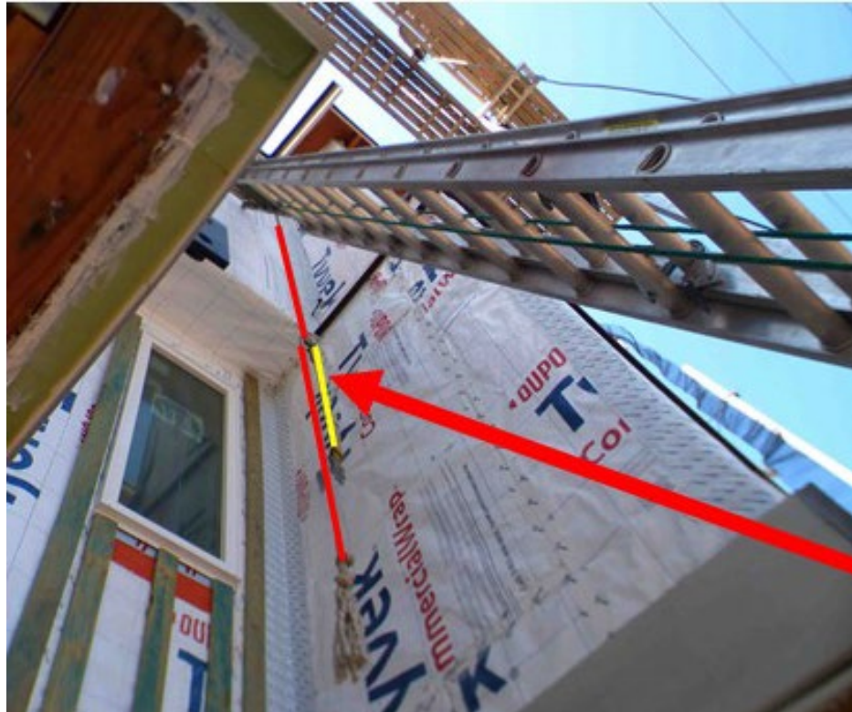
Photo 2. Rope grab lifeline (in red) with connector (in yellow) that worker did not use, as he was not wearing his full body harness. The scaffold walkway and workbench are visible in the top center of the photo.
