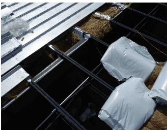
Edge of low-pitch metal roof from which the roofer fell.
