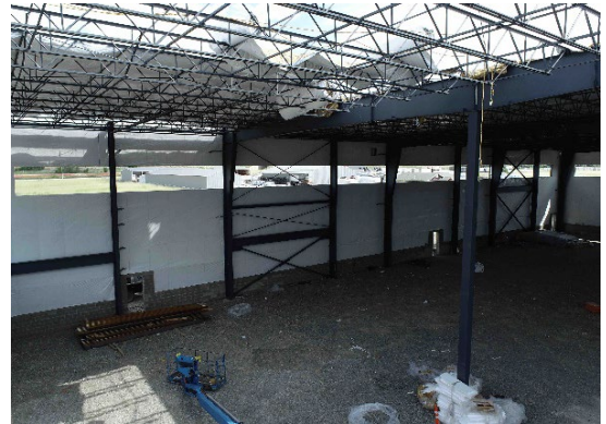
Inside of warehouse where the roofer fell 33 feet from the roof onto the gravel floor.
