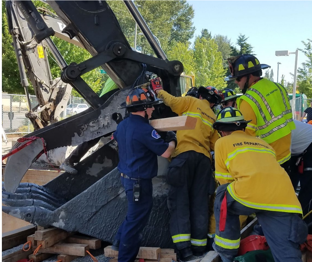
Photo 6. Rescue workers using bracing to prevent the bucket from shifting and other tools while trying to free the spotter's fingers from the coupler.
