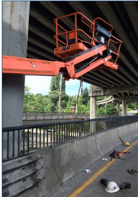
Incident scene showing the aerial lift after being struck by a truck.
