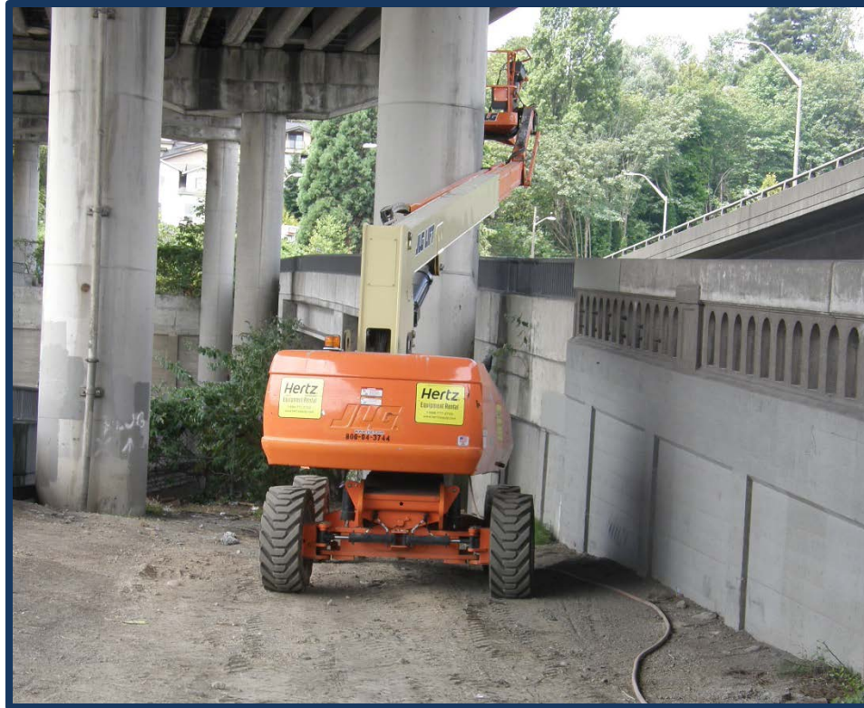
Incident scene showing the aerial lift positioned in a median under the bridge.
