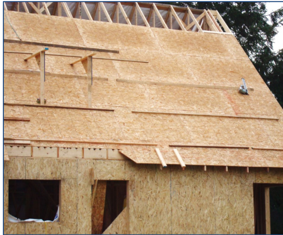
The 12/12 pitch residential roof where a framer was installing sheathing when he fell 18 feet, landing on concrete. He was not using fall protection.
