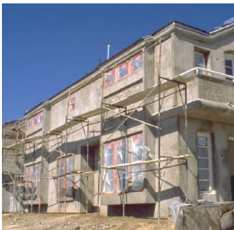
Scaffold needing guard rails
