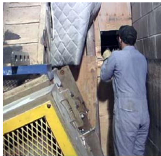
The new way: Now grinder blades are only lifted once, on the other side of the hatch
