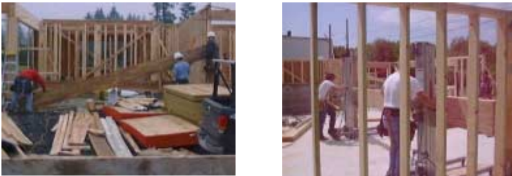
Figure 2. The traditional method for lifting beams weighing 500-800 lbs is shown on the left. Using crane lifts to lift and position beam, eliminating the Hazard Zone lifting risk factor, is shown on the right. Equipment rental cost was $88 for two lifts.
