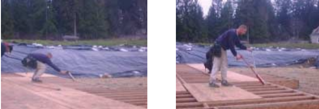
Figure 1. Gluing joists during deck installation (left) can contribute to the amount of back bending. The modification (right) uses commercially available extended gun ($50 retail). A handle was added to the gun to reduce hand/wrist fatigue (<$10 for parts). Job times were the same between two methods. Handle extensions are also widely available for nail gun and screw guns with auto-feed.
