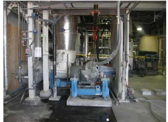
Boric acid evaporator recirculation pump.
