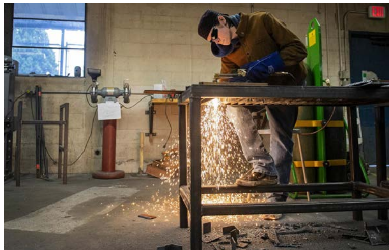
Mark Morris student Gregory Trukken cuts a piece of steel with an oxy-acetylene torch in the pre-apprenticeship program at Mark Morris High School Friday morning.
