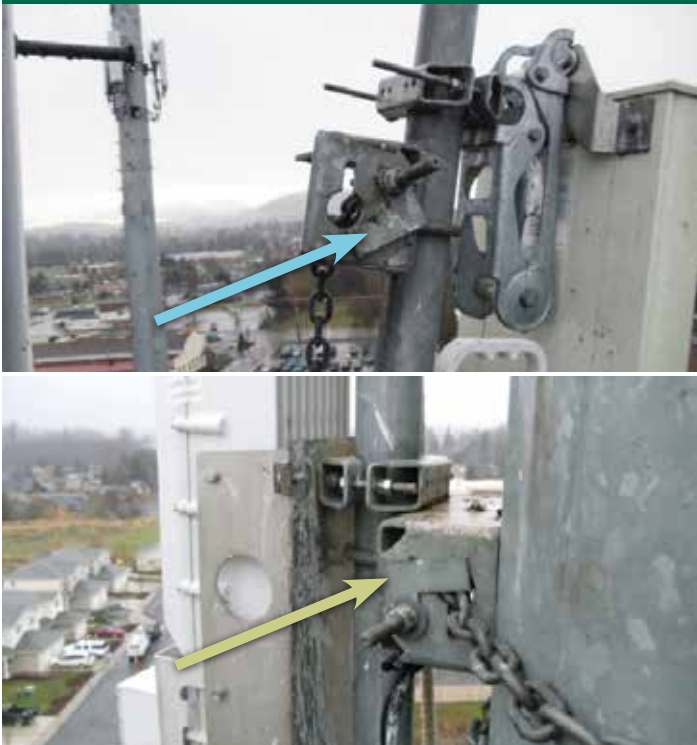
The green arrow shows the correct installation of a chain mount box. The blue arrow shows the chain mount box that failed (it was installed upside down.)
