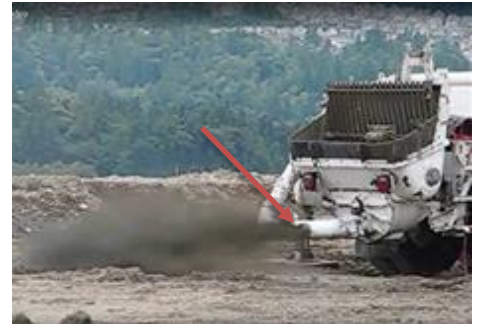
Blowouts can occur suddenly before you have a chance to react. Better to protect workers from blowouts now before someone gets hurt.
