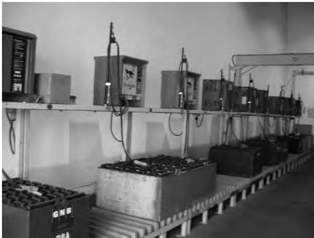
Batteries and battery chargers for electric forklifts.
