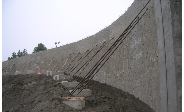
Retaining wall before plywood forms were placed and concrete caps were poured.
