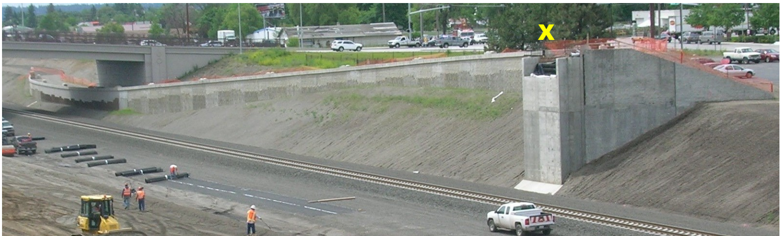
Retaining wall where the carpenter was removing plywood forms from the concrete caps on the top of the wall on the day of the incident. The "X" indicates the area where he was working when he fell.
