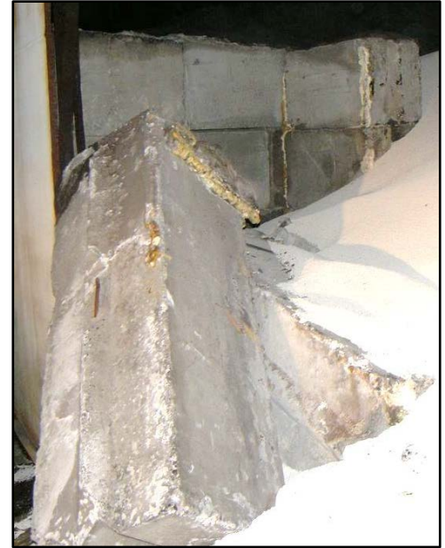
Photo of fallen ecology block against tank wall
