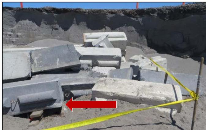
Collapsed ecology block wall. Arrow indicates block that struck victim
