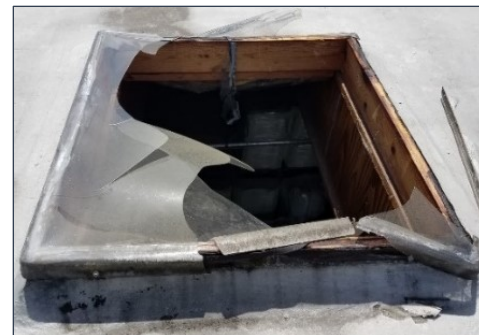
Skylight the roofer fell through.
