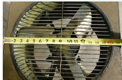
Photo 3: Closer view of the fan blade and grate. The gaps in the grate are approximately 1/2 inch.
