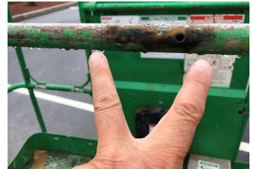
Location where electric current made contact on railing of boom lift basket after arcing from a power line.
