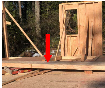
Section of the fallen wall where the crew leader was working.
