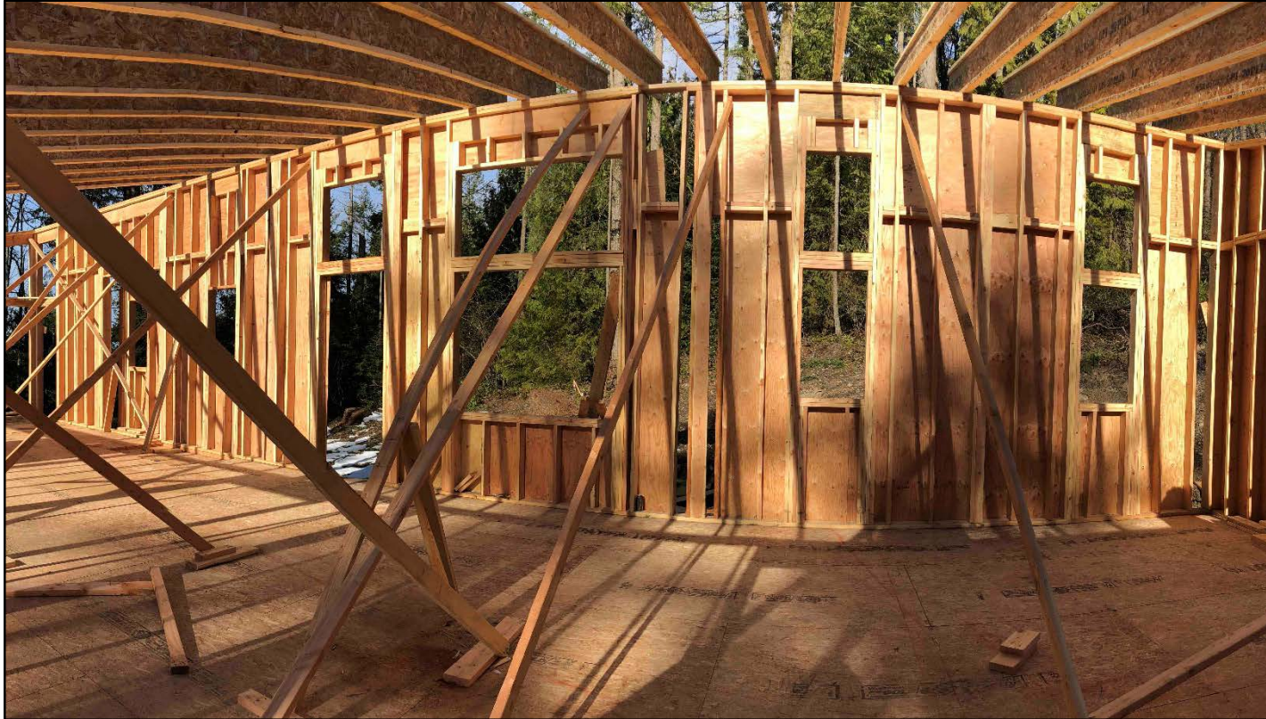
Photo 4. Panoramic view of wall that had fallen. The wall was approximately 43 feet long by 13 feet high.
