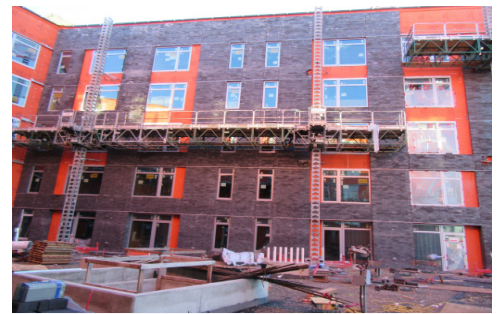
Photo 1: Area where the incident occurred. The scaffold was raised to the fourth story when the plank fell.
