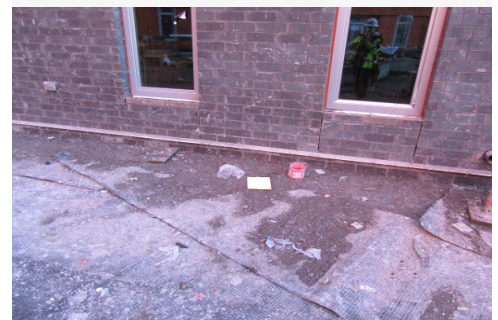
Photo 3: The worker was cutting waterproofing material when he was struck by the falling plank.
