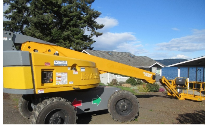
Incident scene driveway of residence with boom lift that workers were using to limb trees.
