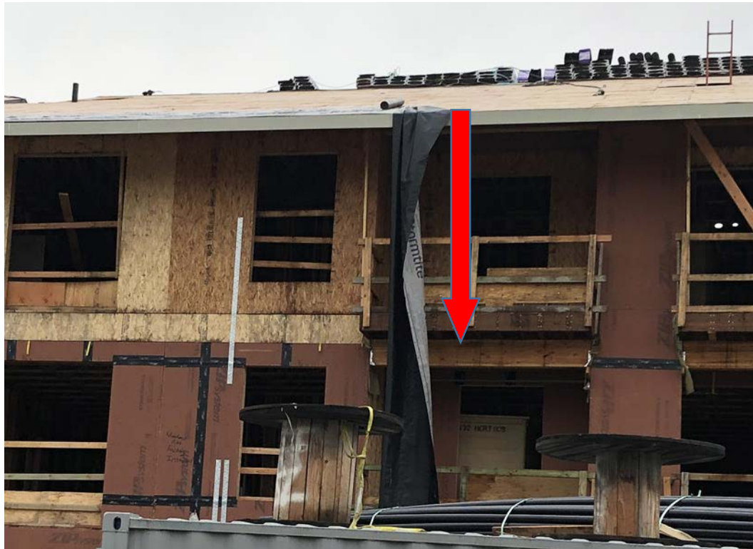
Photo 2. Incident scene showing the location where the roofer fell 30 feet from the roof.
