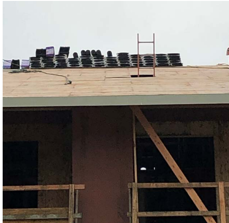
Photo 1. Roof location from where the roofer fell. He accessed the roof's deck by a ladder from the building's third story. Roofing material is shown near the roof's ridge.
