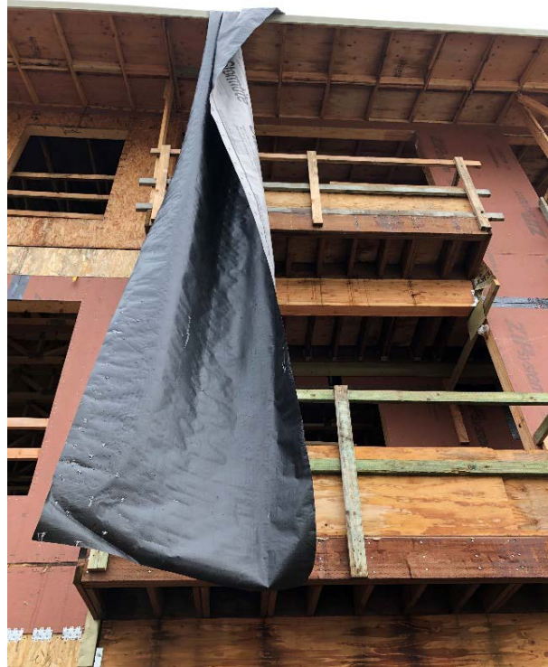
Photo 3. Roofing underlayment he attempted to grab on to as he was falling.
