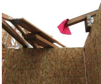
View of the wall from which the laborer fell. A roof truss is marked with a red flag.
