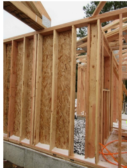
Framed wall from which the laborer fell nearly 10 feet.
