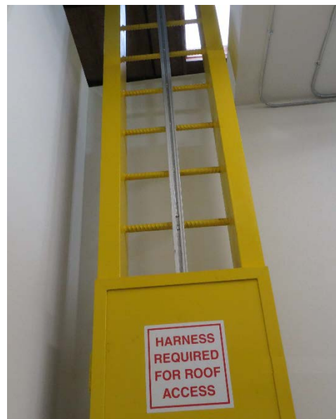
Access point for fixed ladder used to access warehouse roof. At the time of the incident there was no sign indicating that fall protection was required to access the ladder.
