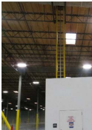
Roof access fixed ladder inside warehouse.
