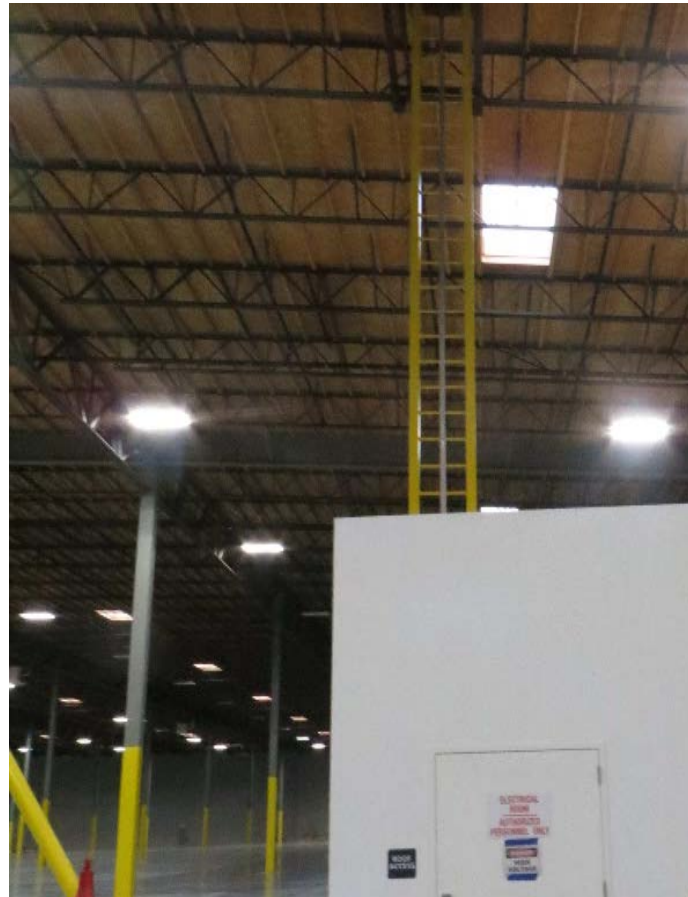
Photo 1. Roof access fixed ladder inside warehouse. Access to the ladder was located inside the electrical room.
