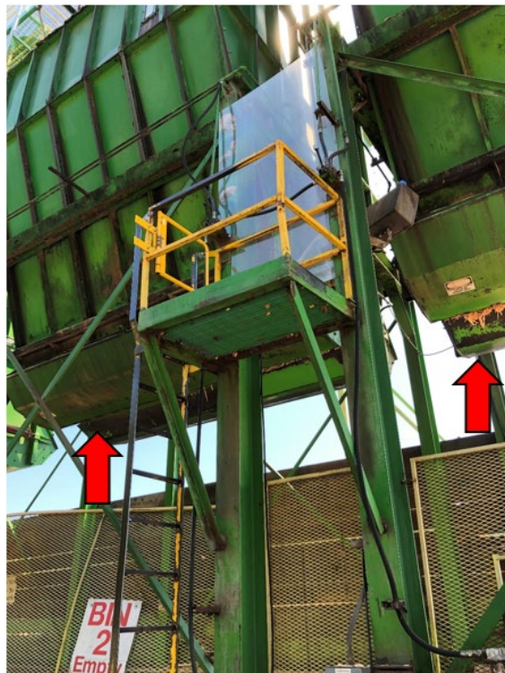
Photo 9: Bin control platform with ladder that truck drivers used to access hydraulic levers for bottom gates that released woodchips into the trailer. Arrows point to the gates.
