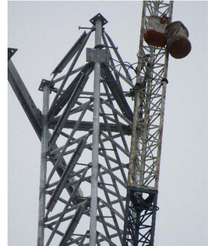
Tower from which the climber fell with the smaller triangular gin pole suspended in the front.
