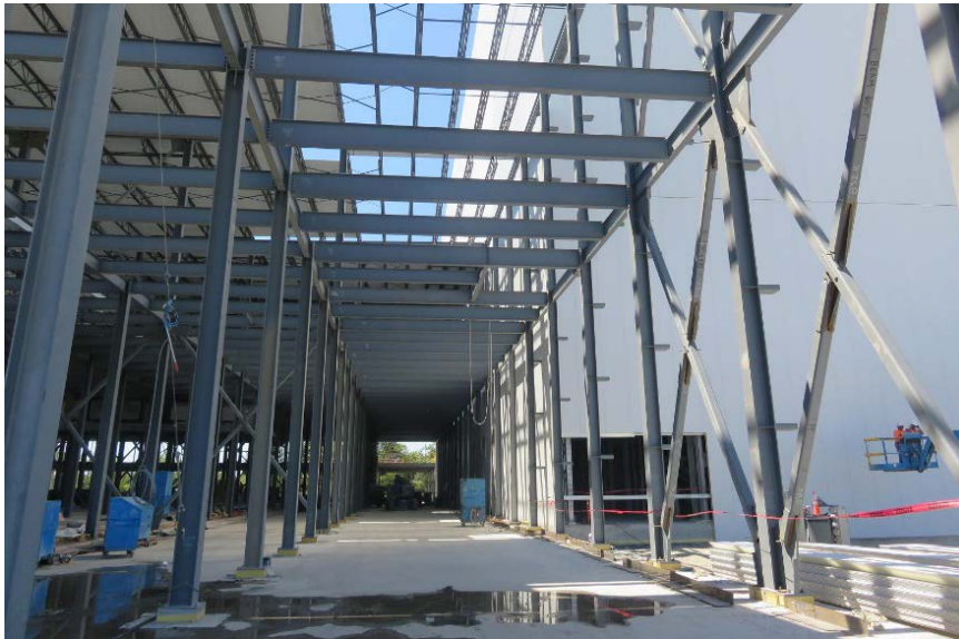
Photo 2. Interior view of incident scene at the cold storage facility under construction.
