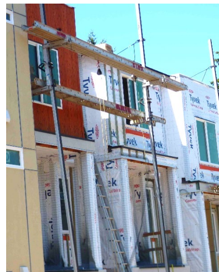
Unguarded pump jack scaffold from which the siding installer fell 23 feet.
