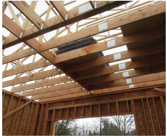
View through the unfinished floor of the room above the garage. The leading edge of the floor is on the right and the OSB sheathing is stacked on floor joists.
