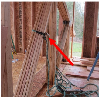
Example of how crew tied-off lifeline ropes to roof trusses.
