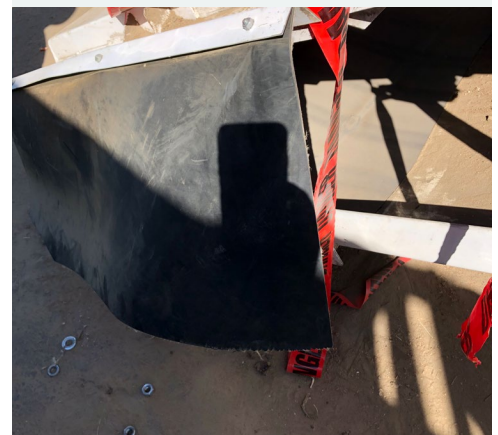
Roller guard that the injured worker lifted to access the conveyor belt.
