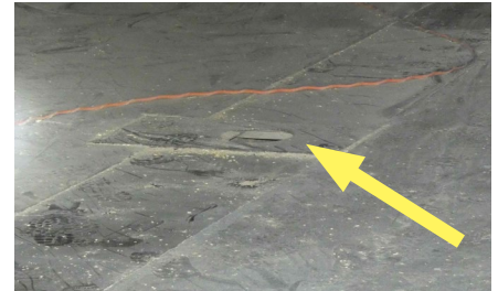
Incident 1: Arrow points to the auger hole the worker stepped in while sweeping in dark, dusty conditions.
