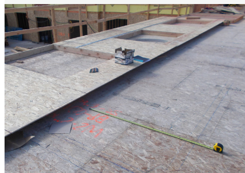
The tape measure shows the approximate place the worker was standing while cutting the board.
