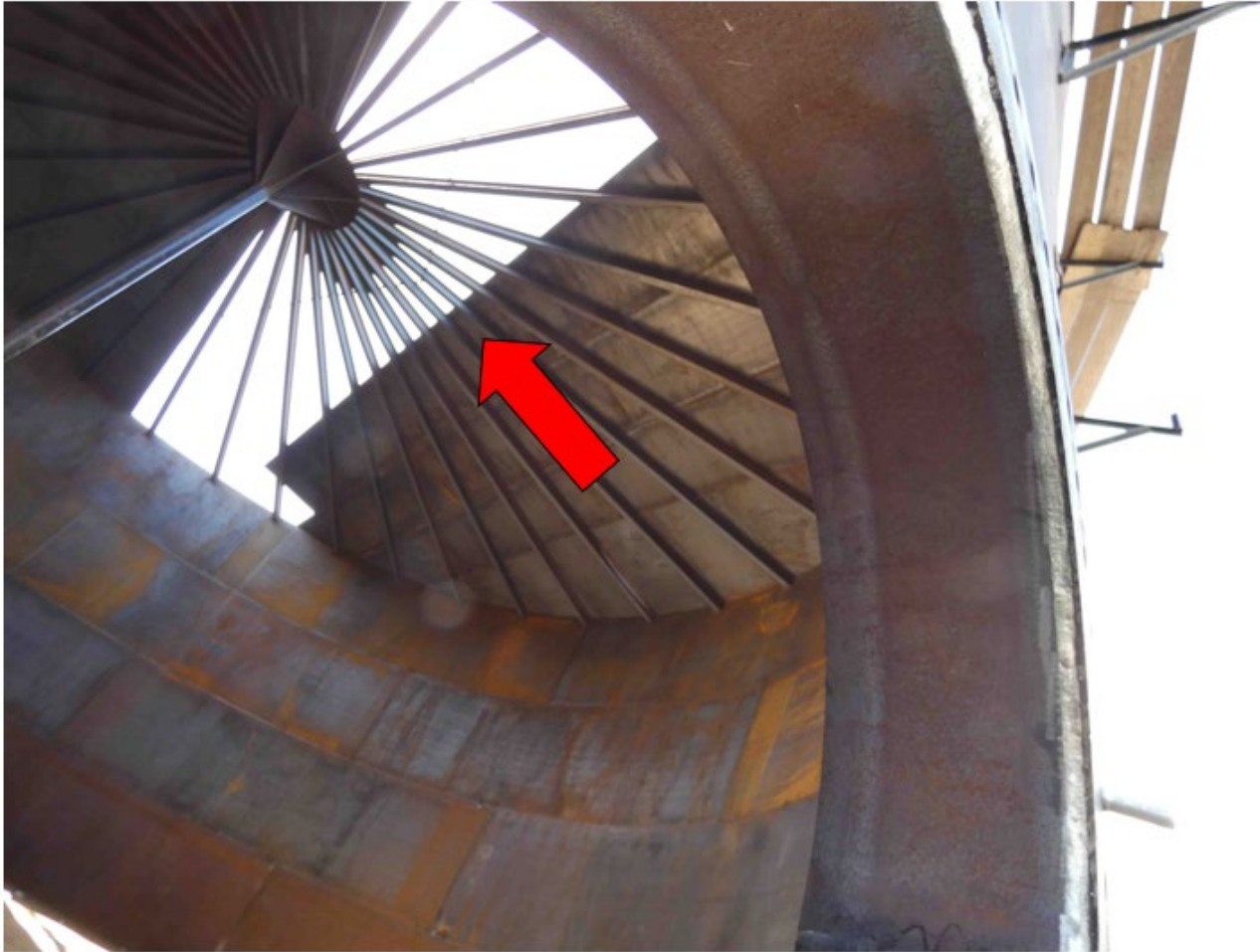
Photo 3. Alternate view of hole in tank roof where the welder fell.
