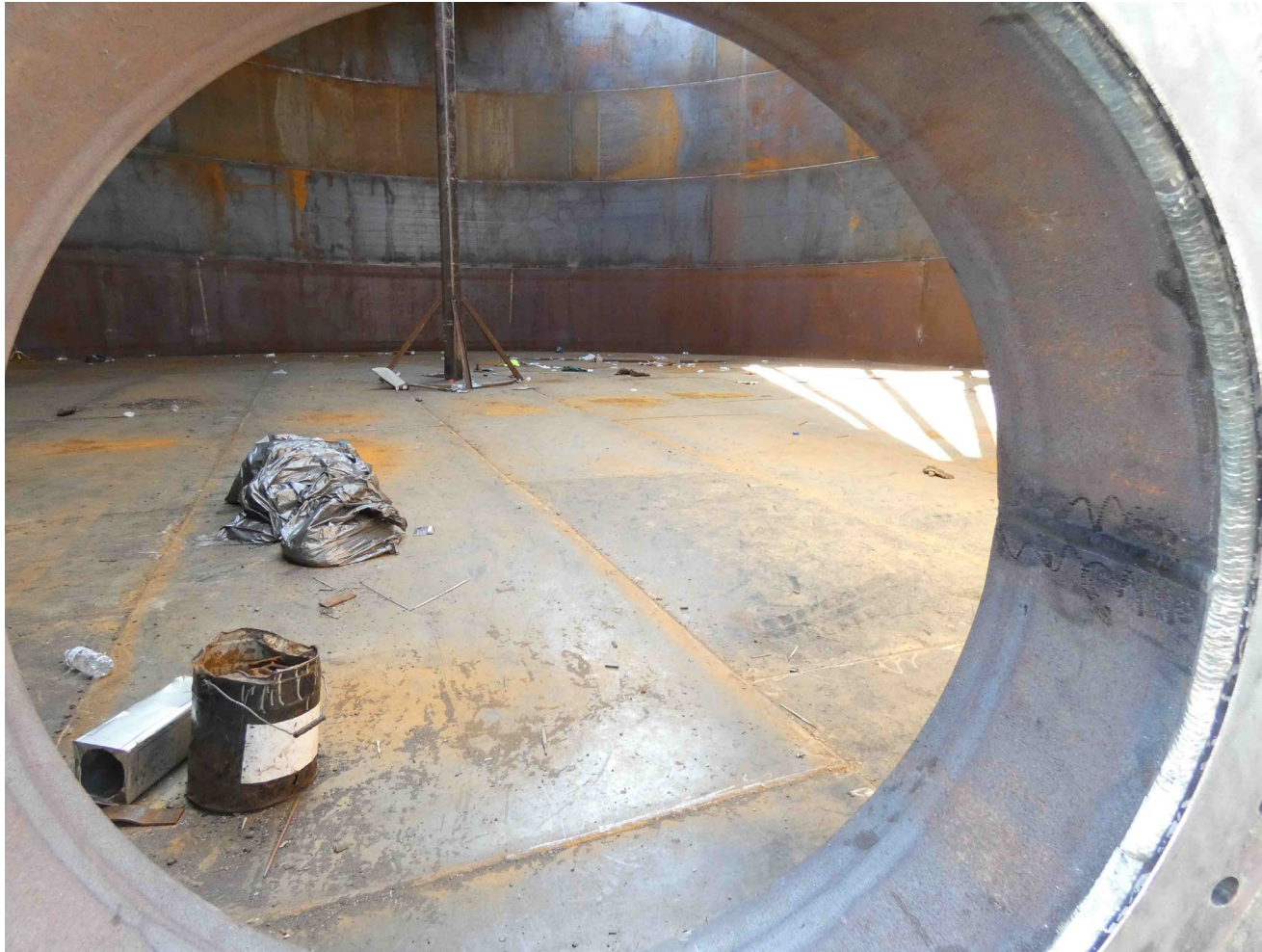
Photo 4. Floor at base of tank where the welder landed.
