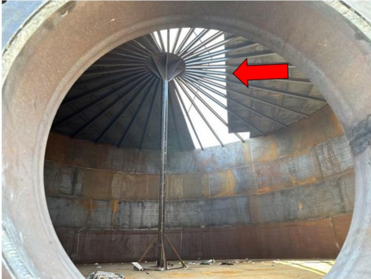
Photo 2. Hole in top of tank roof where the welder fell through.
