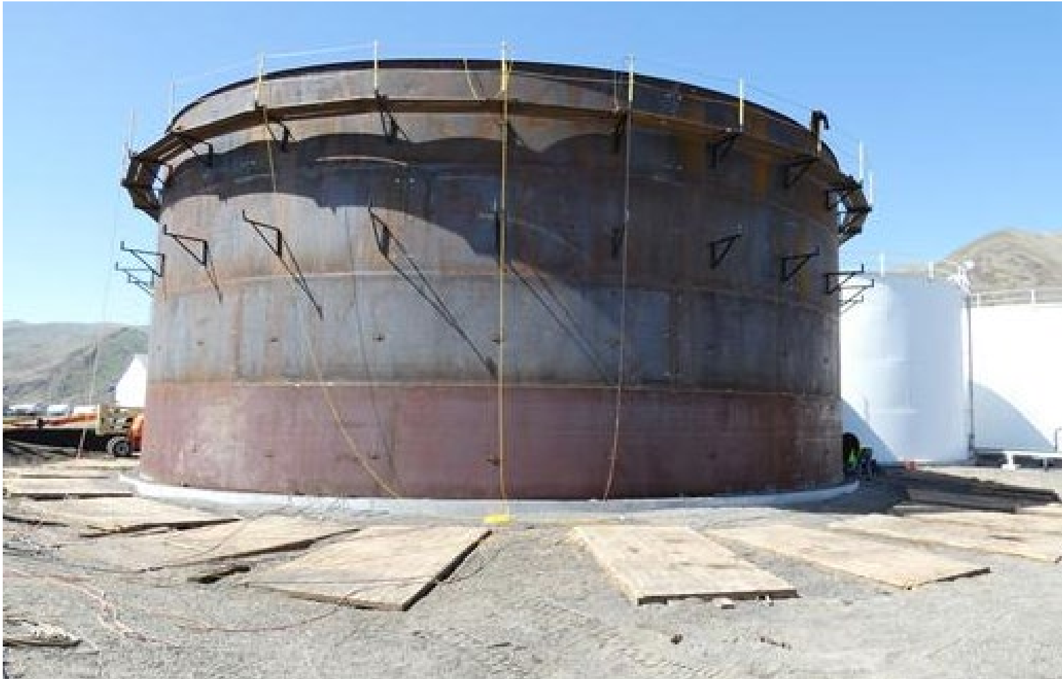
Photo 1. Storage tank at incident site.
