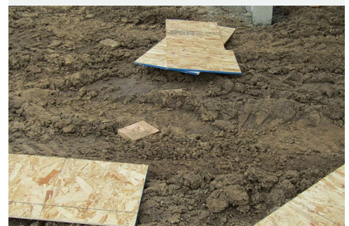
Figure 3: The frozen ground where the worker landed after the fall.
