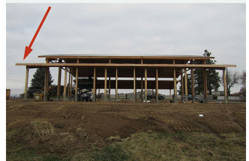
Figure 2: Area on barn roof where worker slipped and fell after he unhooked his fall protection (red arrow).
