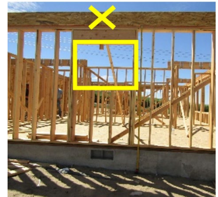
Framer fell from rim joist (x) above window opening to floor deck.
